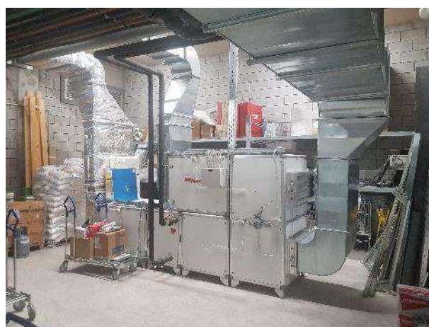
Air Handling Unit (AHU)
