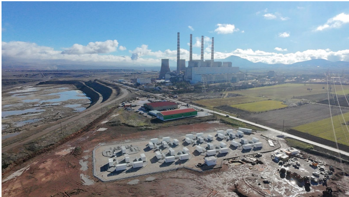
Figure 4: Battery array of the Ptolemaida IV Electrochemical Energy Storage Station. The Kardia Power Plant can be seen in the background, along with the location of the lower reservoir of the future pumped storage station.
